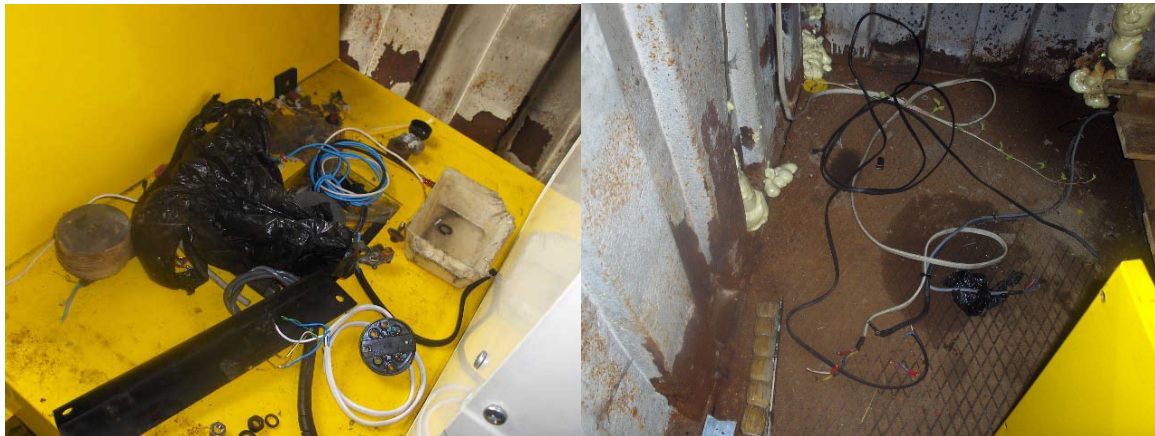
DAMAGED AND MISSING RADIO EQUIPMENT
